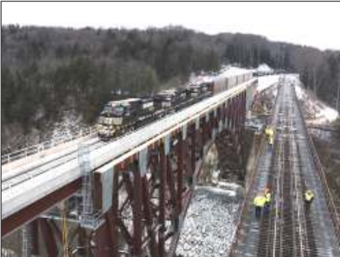
Norfolk Southern C44-9W No. 9345 leads train 36T, a Buffalo, N.Y., to Allentown, Pa., manifest train on a new steel arch span on Dec. 11. The arch replaces an iron truss bridge built by the Erie Railroad in 1875 and shown on the right.
