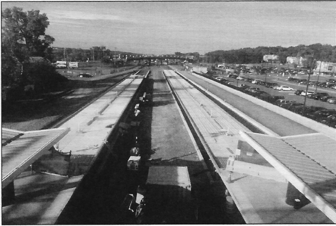
New platform construction at Albany-Rensselaer Station, from Herrick Street Bridge looking north towards Amtrak maintenance facility and yard.
