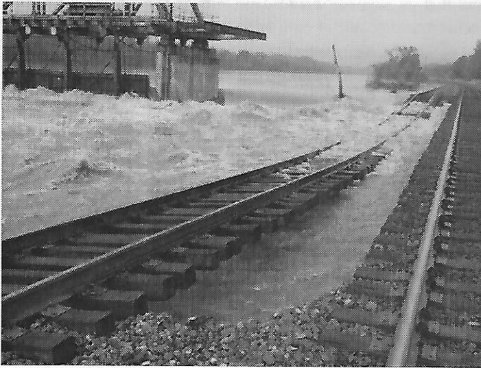
Washout west of Fonda, NY on CSX's Mohawk Sub-Division.
